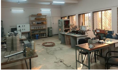
High Voltage Lab
